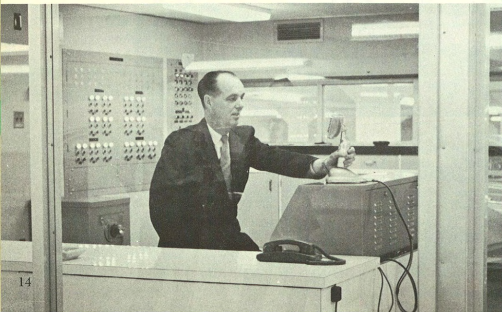
The underground Civic Garage is operated from a central control booth equipped with public address system.
