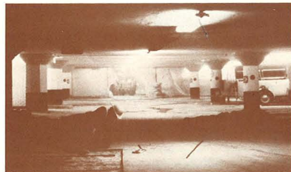
Work being undertaken to repair floor slab at municipal carpark 36, the Nathan Phillips Square Underground Garage
