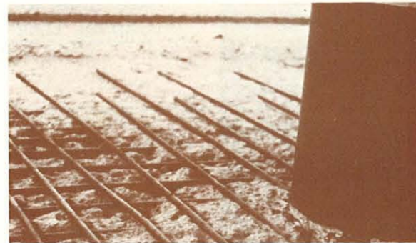
Damaged concrete removed to expose reinforcing bars
