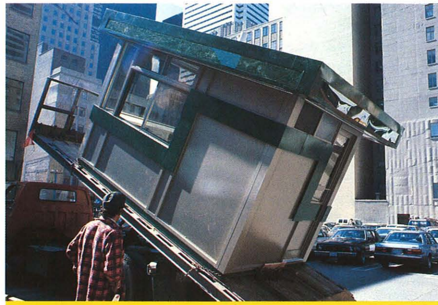
A pre-fabricated cashier shelter is set into place at the Temperance Street surface carpark. These shelters are designed to be portable so that they can be moved to new locations with the closing and opening of carparks.
